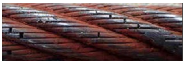
Fig.: Internal corrosion - 100% discard
