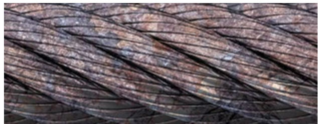
Fig.: Medium corrosion, 40% - 60% severity
